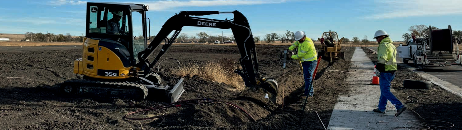
This fall, the Kimball crew worked to bring power to a future housing development in Fort Thompson.
