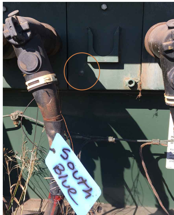
Left: A bullet dented portions of the electrical equipment inside the underground cabinet that FEM Electric Association crews found damaged by gunshots.
