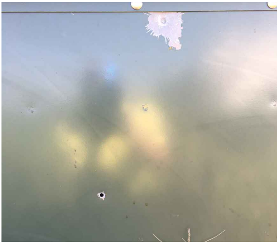
Left: Crews at FEM Electric Association in Ipswich, S.D., found bullet holes in an cabinet this fall. The damage from the bullets did not cause immediate outages, but did weaken the equipment.
